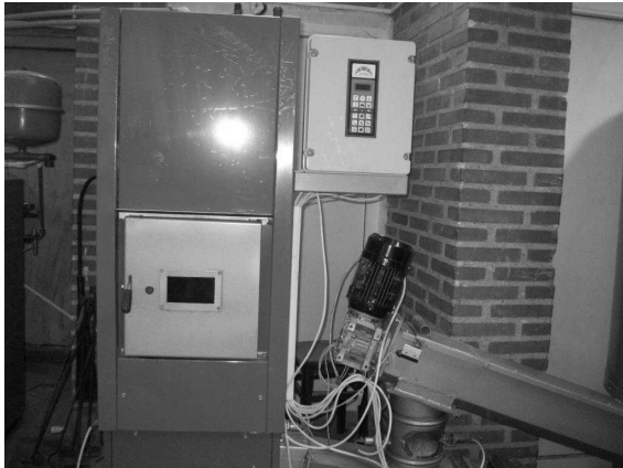
Fig. 7. The 40 kW thermal boilers view
